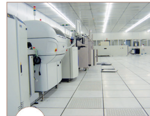
1000 class clean room
